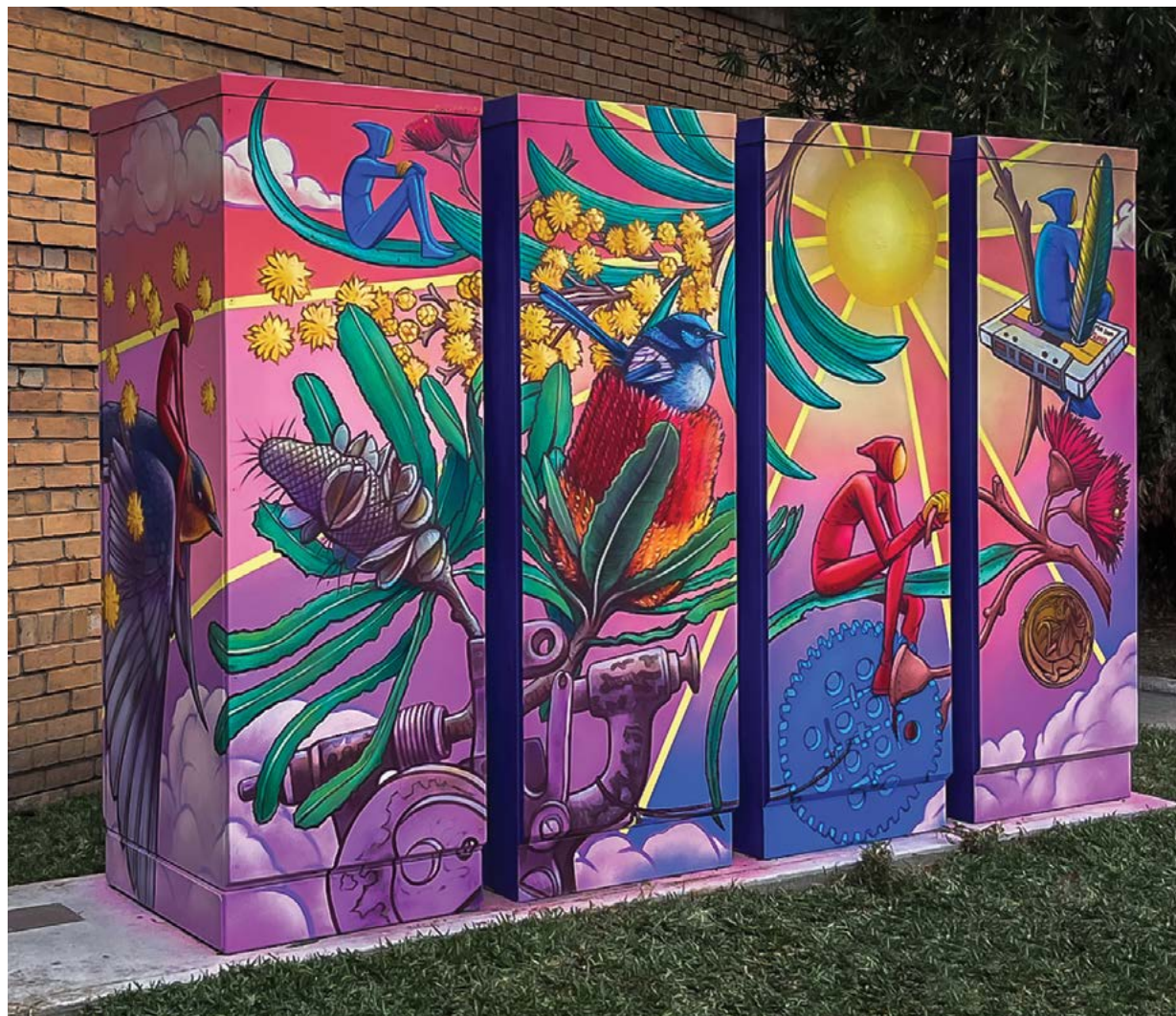
CitiPower partnered with the Yarra Energy Foundation to install a 284kWh community battery in Fitzroy North in 2022. This was the first inner-urban battery in Melbourne and supports an estimated 200 homes.
