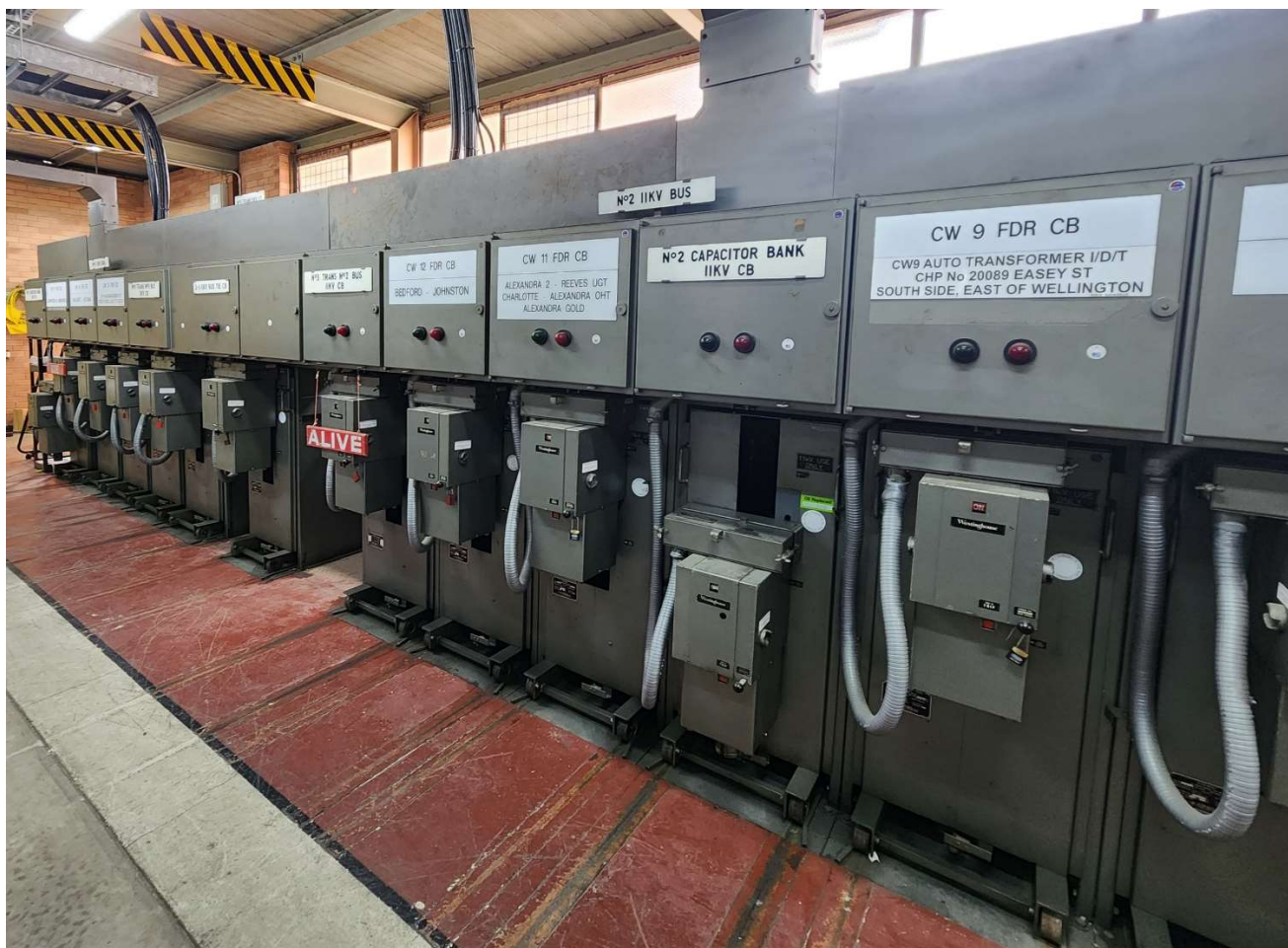
Figure 7: Existing 1960's Email J Series Indoor Metal Clad Switchboard
