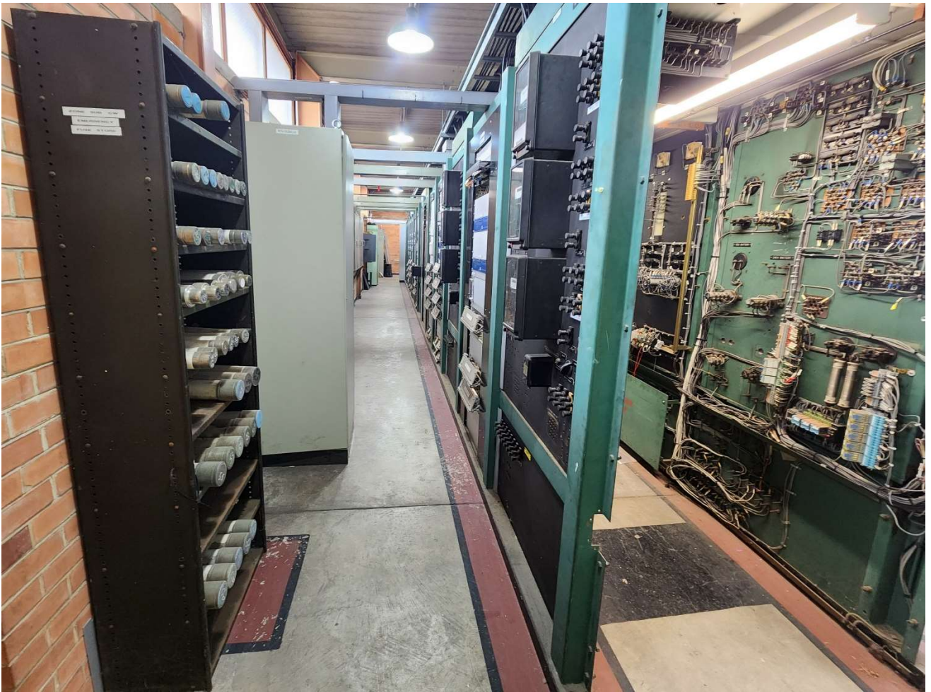
Figure 8: Existing 1960's Electromechanical Protection and Control Relays and Secondary Asset Panels
