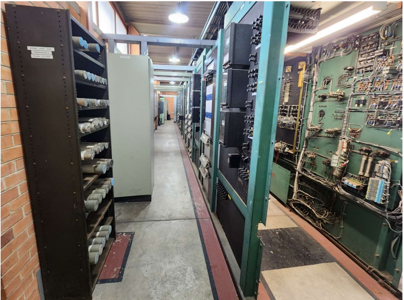
Figure 7: Existing 1960's Electromechanical Protection and Control Relays and Secondary Asset Panels
