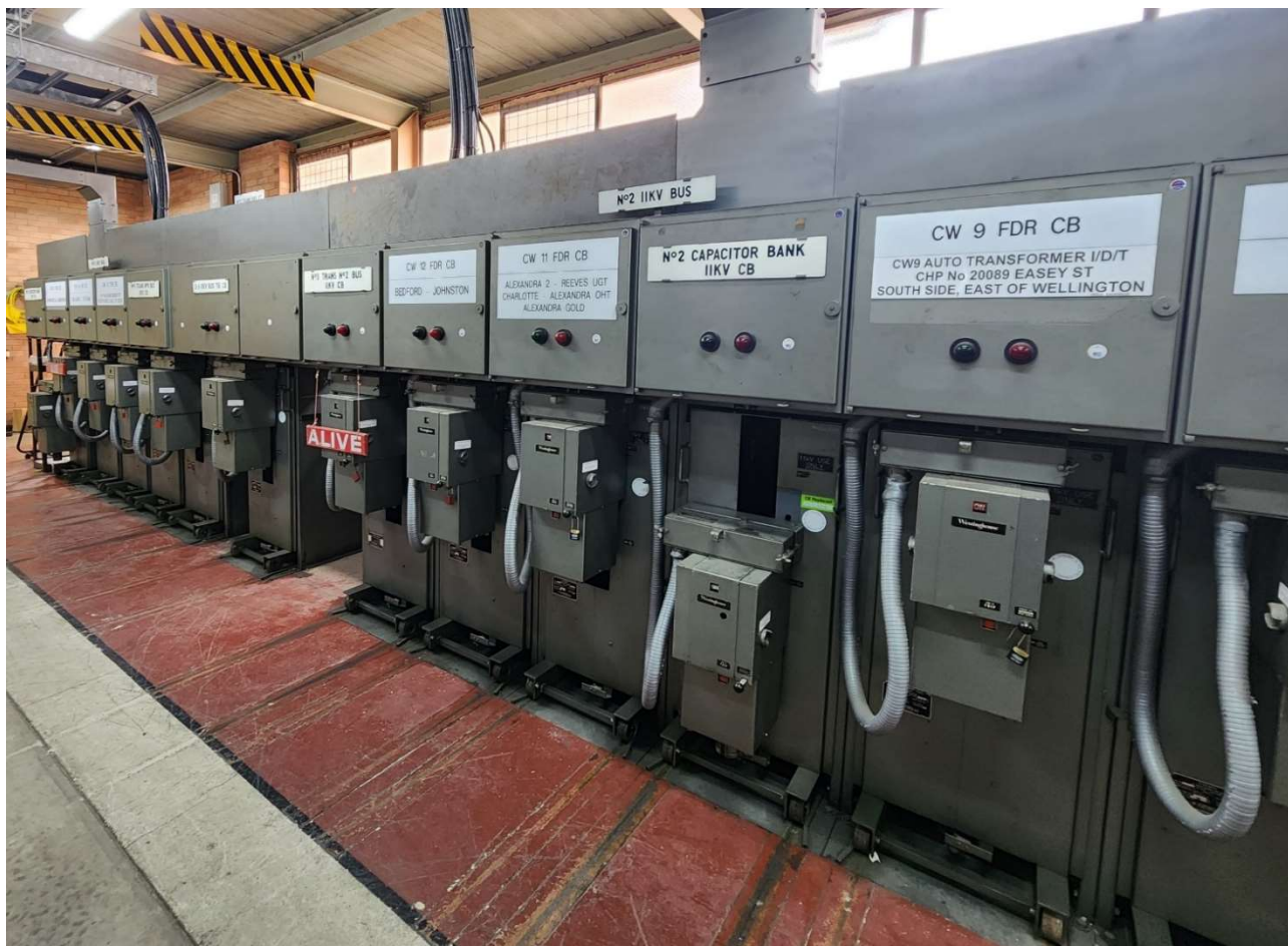
Figure 6: Existing 1960's Email J Series Indoor Metal Clad Switchboard
