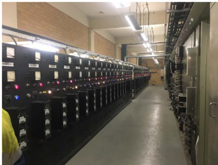
Existing early 1970's electromechanical protection relays
