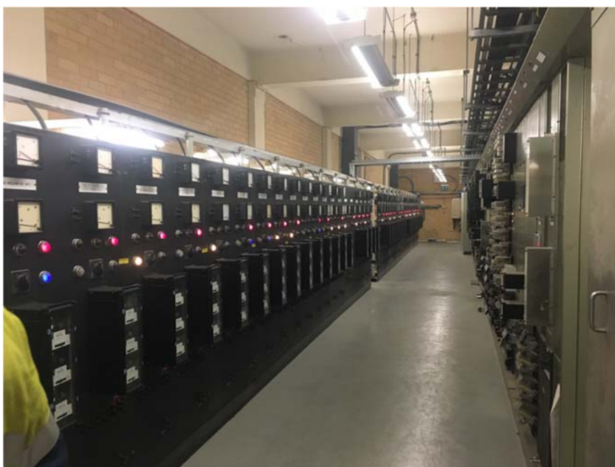
Figure 7: Existing early 1970's electromechanical protection relays
