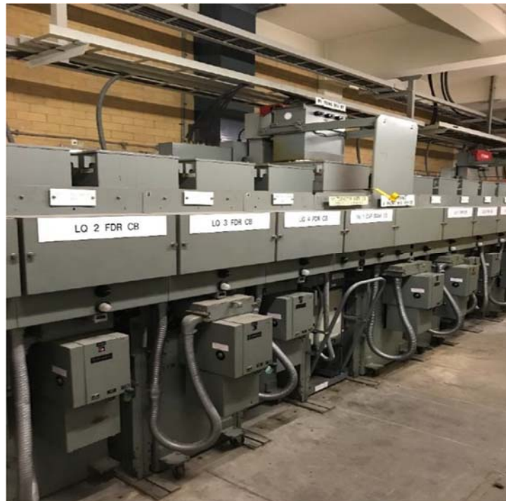
Figure 6: Existing Email HQ compound filled double bus switch board - Bus A shown
